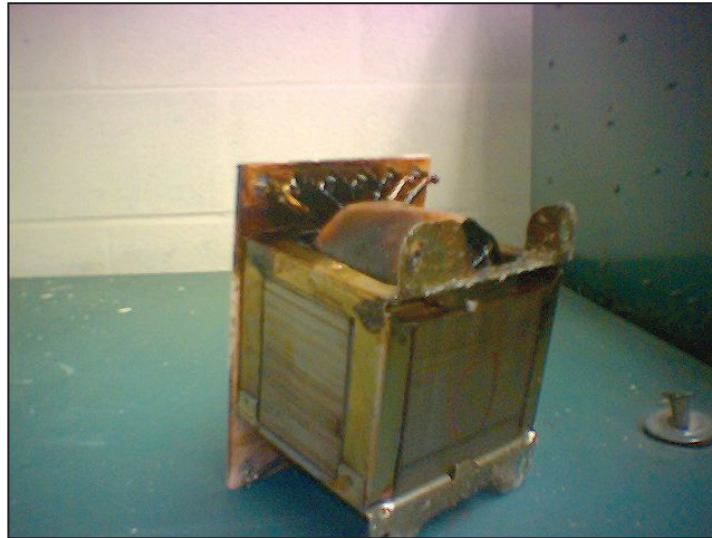
A transformer blew in the Wood Campus center last Monday causing an emergency evacuation of the entire building. PHOTO BY SANDY FORREST
